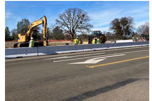
Bass Lake Road at Madera Way Construction photo credit - Tasha Boutselis Camacho
